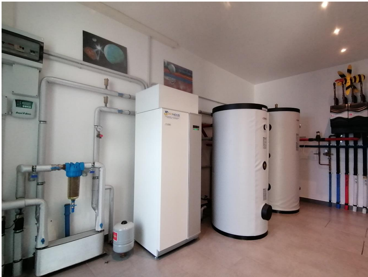
Figure 35 Heat pump NIBE F12345 and buffer tank
